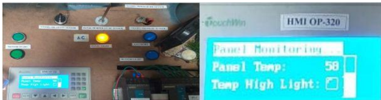
Fig. 7: Panel Temperature Monitoring
